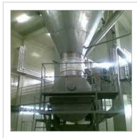
SS Spray Dryers
